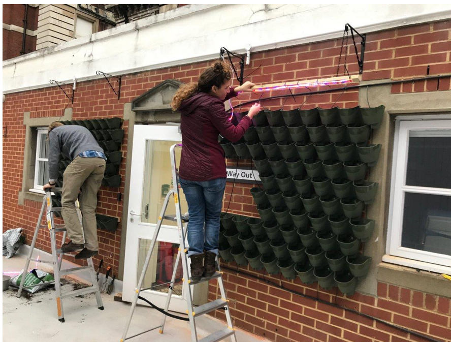
Putting the finishing touches to the LED lighting system at vertical garden Rare Diseases Centre St Thomas' Hospital
